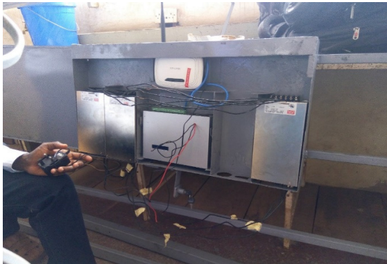
Figure 10: Casing of the router, T-300k controller and the power supply units
