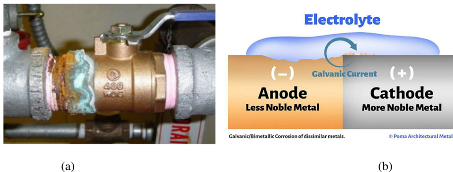
Figure 5: (a) Galvanic corrosion of galvanized piping in connection with bronze valve (Heidersbach, 2018), (b) galvanic corrosion
