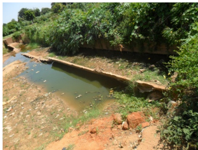
Damaged drainage structure
