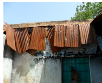
Collapse roof of one of the houses
