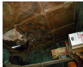
Damaged ceiling due to leaking roof
